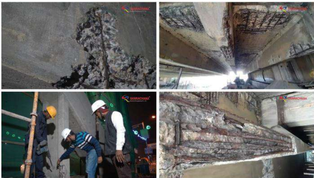
Fig. 2 Spalled portions show exposed and discontinuous rebars in hanger columns, under deck slab and on cross beams
